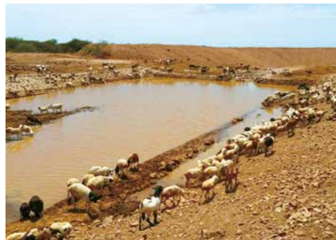
A livestock water point constructed under the project. It supplies water to many head of livestock even during the dry season or drought.
